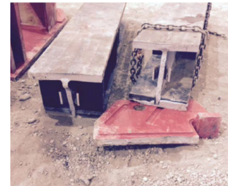
Failed beam parts and snapped off hanger hook
