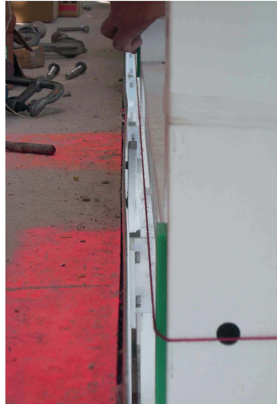
Figure 4.10: Positioning a curtain wall to be assembled in the work in relation to a horizontal line.
