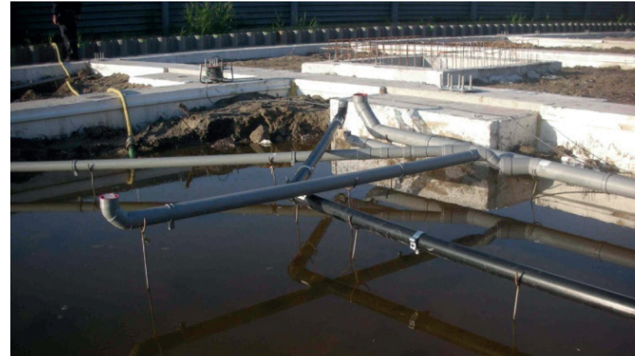
Figure 6.4: The sewer pipelines with metal supports and raising points.
