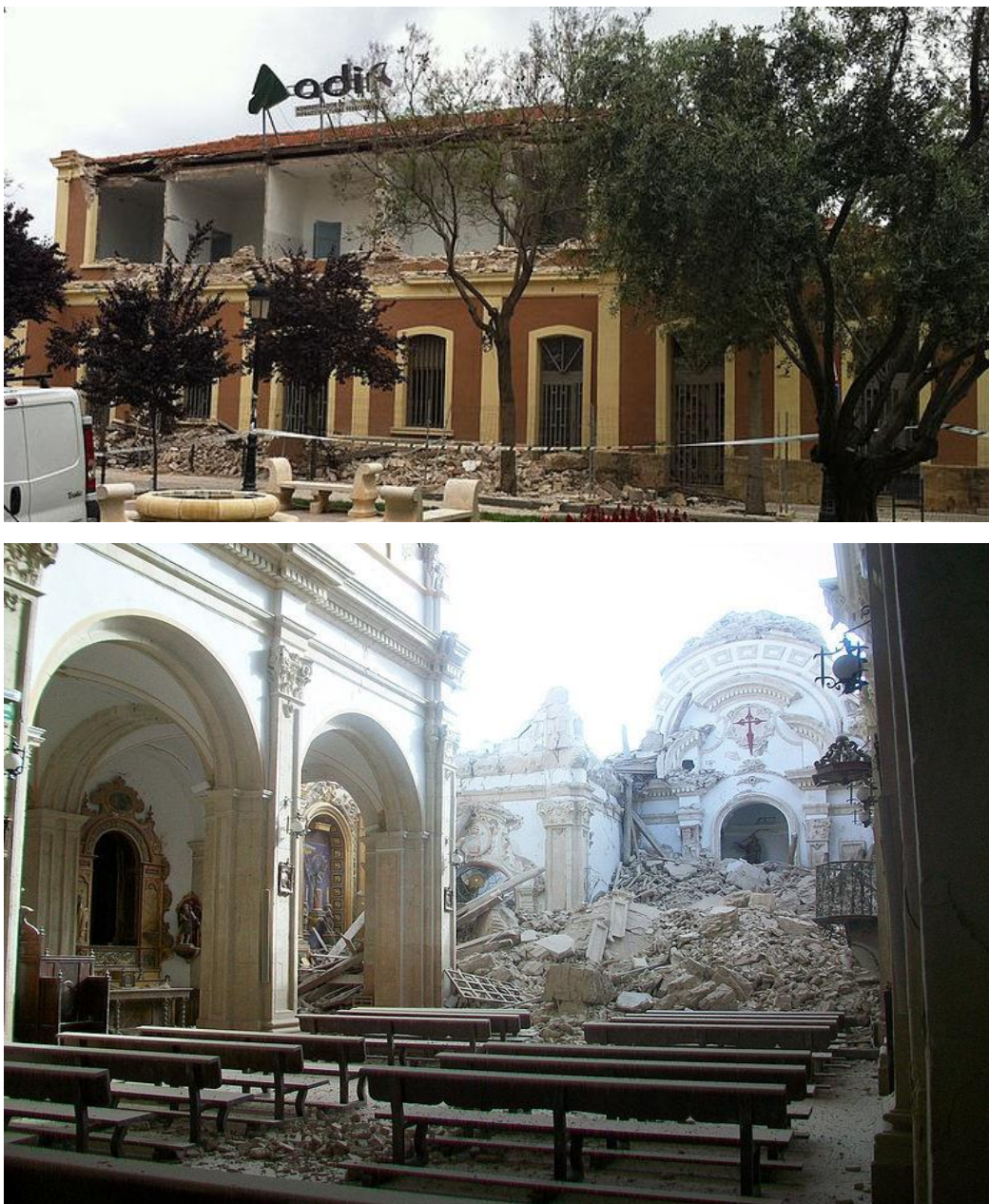
Figure 48 Observations of complete damage and collapse of an old unreinforced masonry church building caused by the Lorca, Spain 2011 earthquake.
